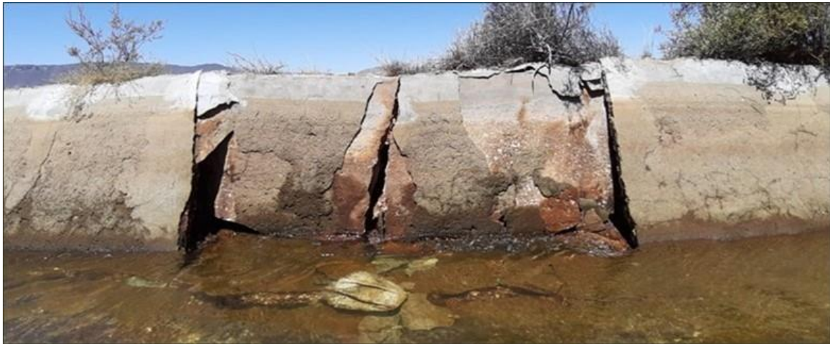
Figure 2-6: Failure in 2019 of the Lower Olifants Canal along the existing main canal
